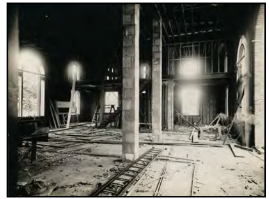
October 2, 1916: Roughing out the interior. Part of the construction progress photo series taken for documentation by the United States Treasury Department.
